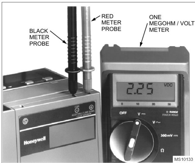
Fig. 11. Measuring voltage flame Signal with 7800 SERIES controls
